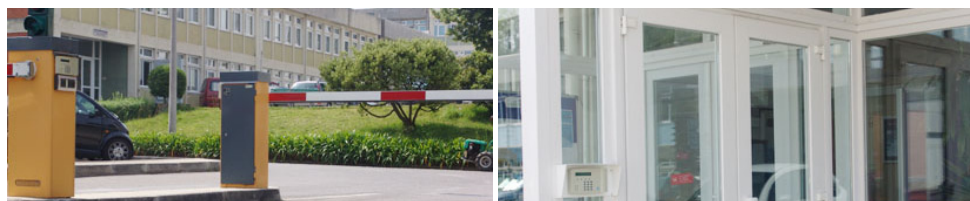
Fig. 7. Campus Access control - Instituto Superior de Engenharia de Coimbra . Installed car park and building access, by a security contractor using HID RFID technology.
